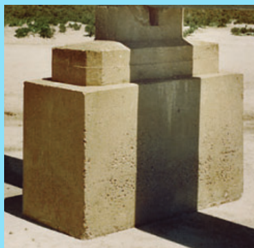
Cast in 1962 to replace damaged chair, with Caltite - condition after 40 years
