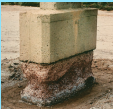
Pipeline support chair cast in 1960 with ordinary concrete after 19 years
